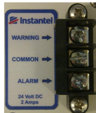
Remote Alarm Terminals
