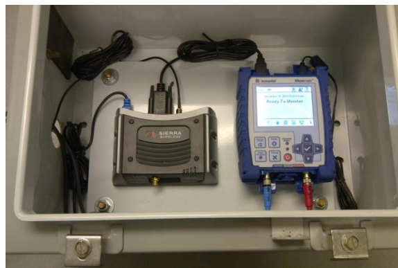
Mounting Panel Installed in the Enclosure
